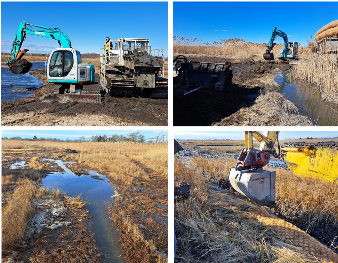
Top Left: Fill material being taken from the newly opened inlet (top left) and being placed on top of coir logs to plug a ditch (top right). Using a low pressure tracked excavator and dump carrier to create the single channel marsh system. Bottom Left: A finished fish micro-pool with a shallow connecting runnel allowing for killifish access. Bottom Right: Coir log being installed to fill an existing ditch.
